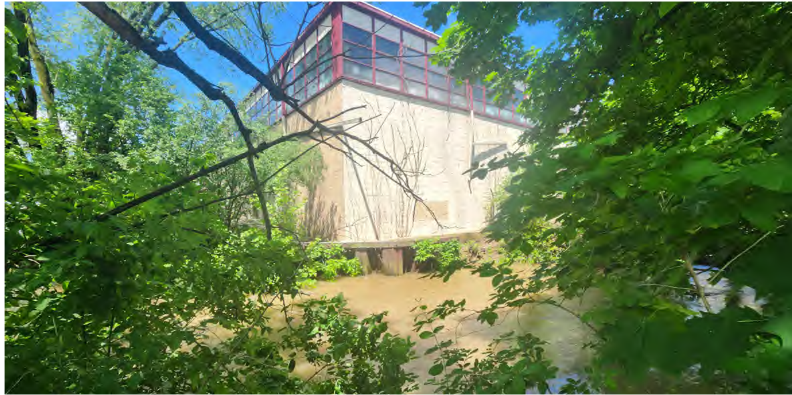
Derelict building constructed into Cedar Creek
